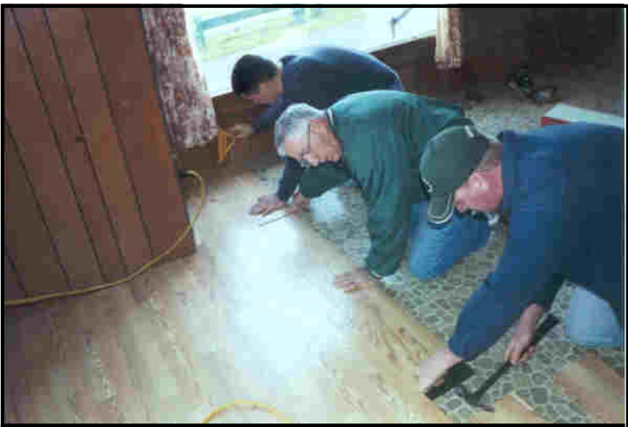
Squadron 396 members Howard Bailey, Ben Desio and Drew Spencer installing a new floor in the Post home.
